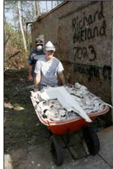
NAU students Stacie Leach and Trent Shumway remove debris from the Breland home in Mississippi.
