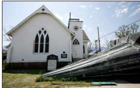
The steeple from the Main Street United Methodist Church in Bay St. Louis, Miss., was moved from the street to the church's front door after it came crashing down during the hurricane.
